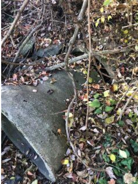
Photograph No. 1 – Separated end section of 36-inch CMP at SWM Basin #3
